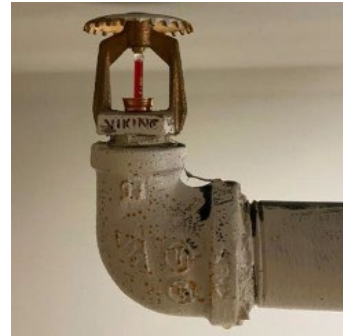
Close-Up of Sprinkler Head
